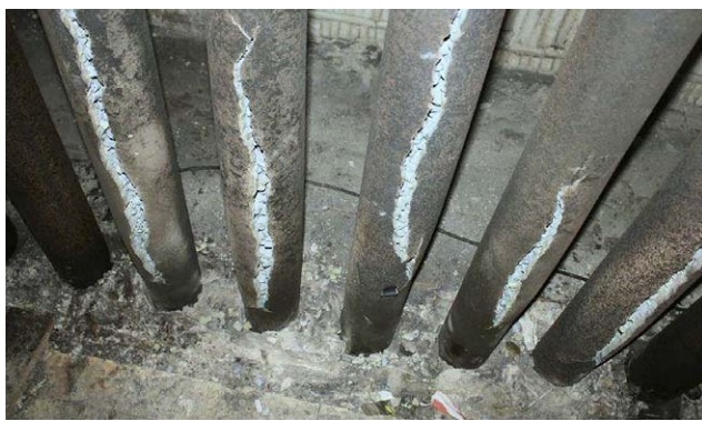
Figure 1. Multiple reformer tubes failed in a side-fired furnace design due to thermal shock/flame impingement.
