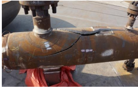
Brittle Failure / Low Temperature
